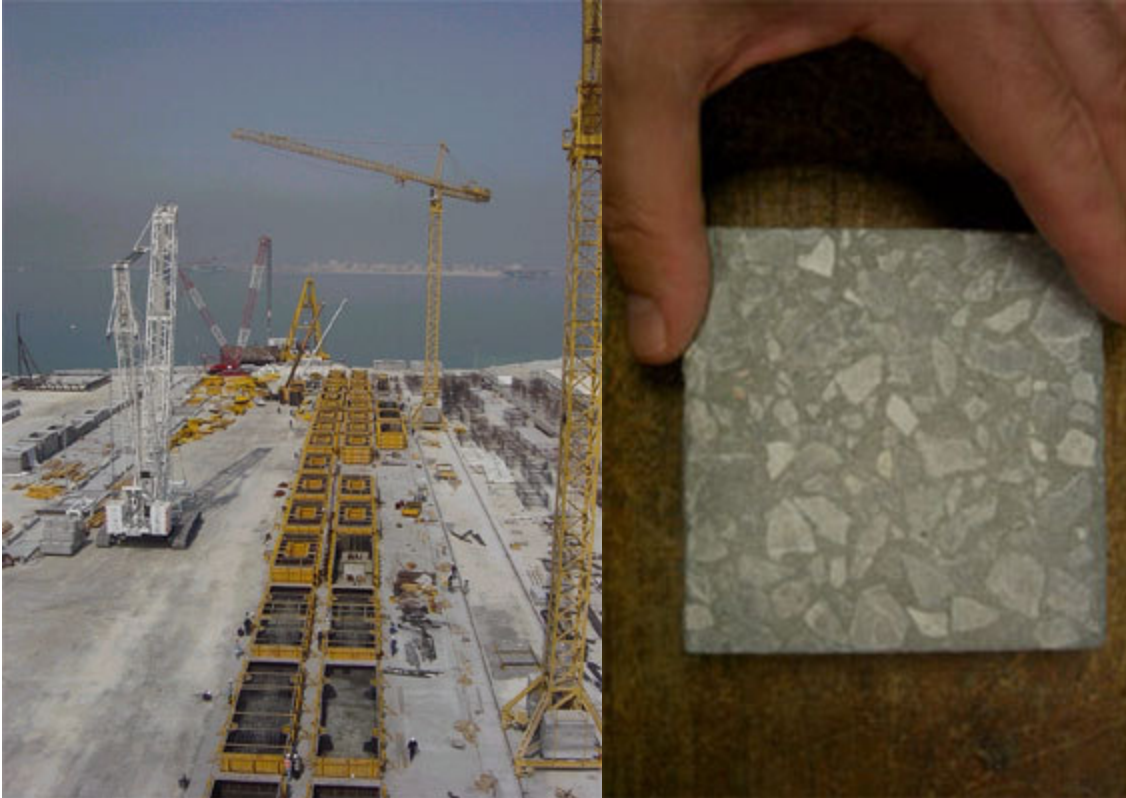
Above left: Concrete works at the port in Bahrain during 2003. Concrete work of the 2.4 km Quay Wall was completed ahead of schedule, with virtually crack-free concrete elements.
