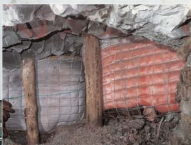
Mine support systems
